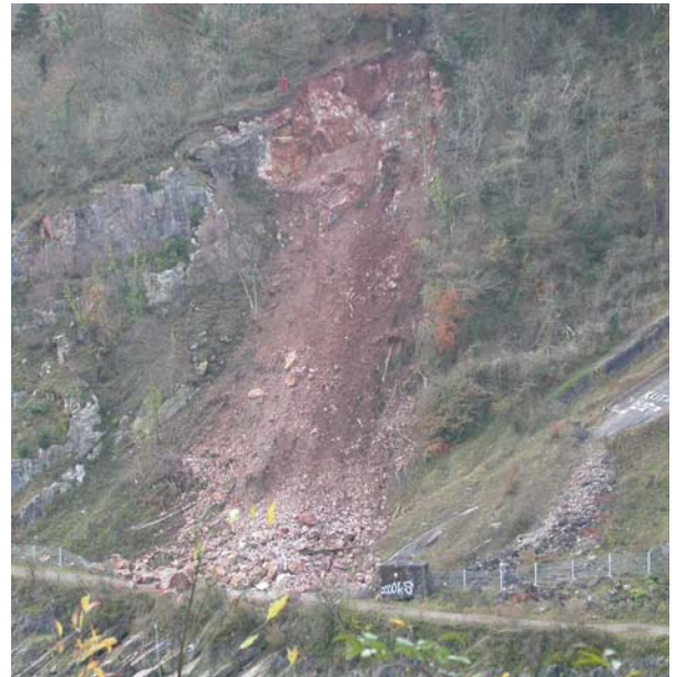
Major rockfall in the Avon Gorge, Bristol. Many tons of rock suddenly crashed down onto a public footpath and cycleway. (Photo by courtesy of National Trust)
