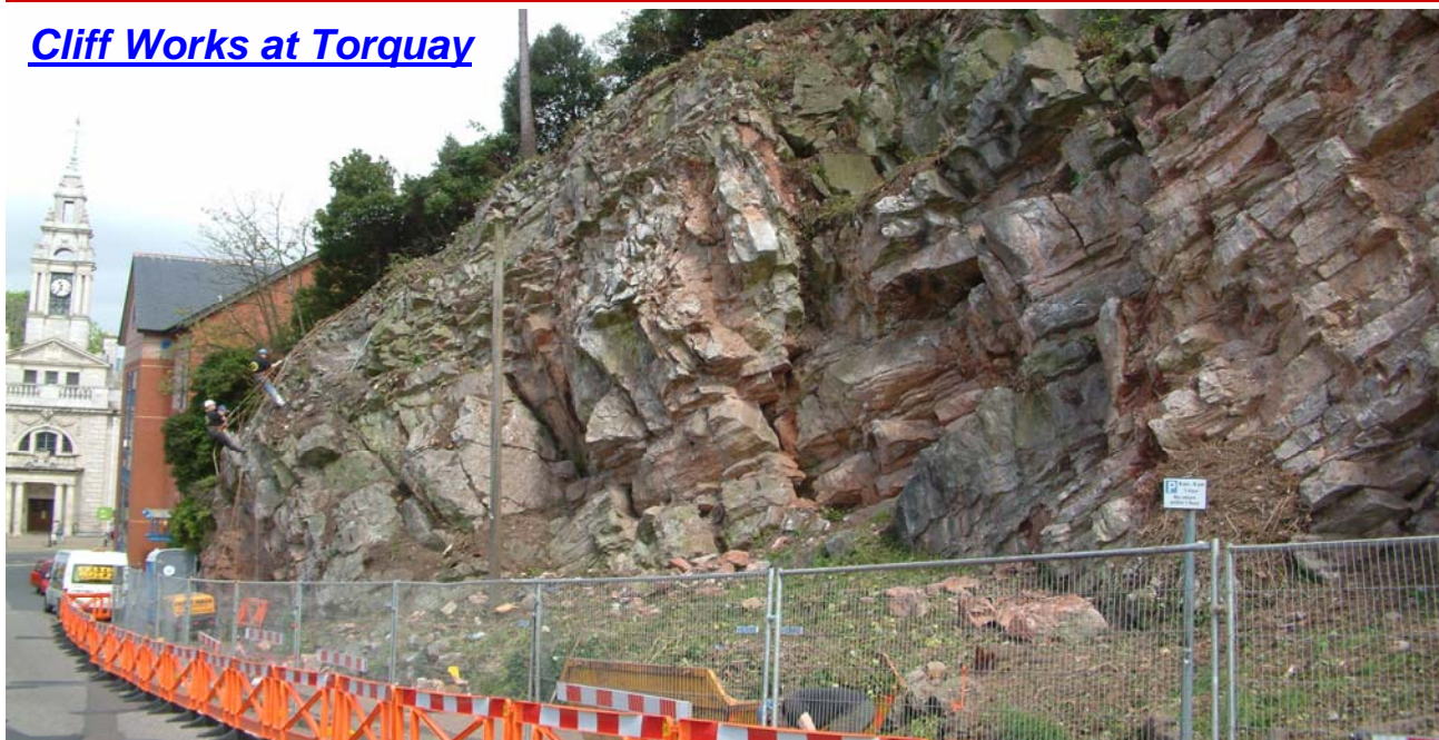
Castle Road, Torquay where the steep rock face in Devonian limestone has been investigated, trimmed and reinforced
